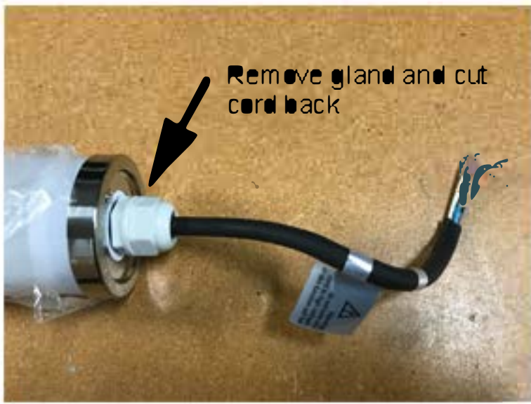
1. Existing fixture has cords coming out of both ends.
